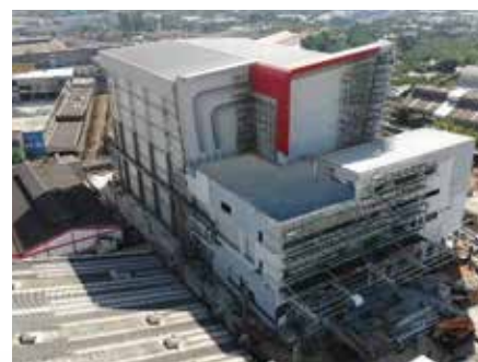
LUCKY UNION FOODS NEW LOGISTICS CENTER ASRS
